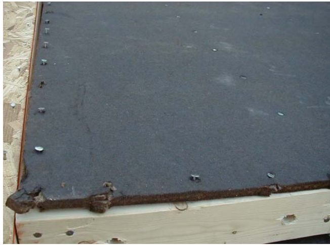
Figure 21: Nail tear-through (fiberboard)
