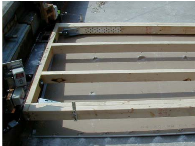
Figure 46: Gypsum nail rip-through along end stud
