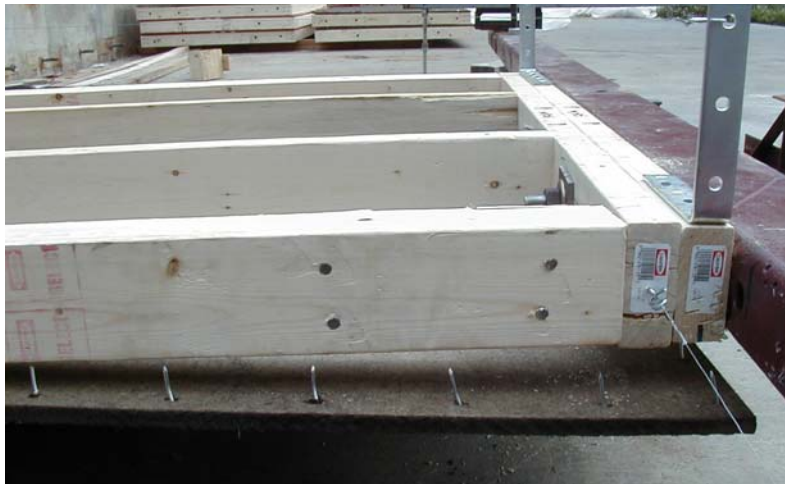
Figure 22: Sheathing-to-framing separation (fiberboard)
