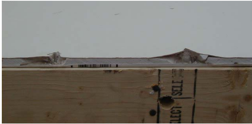
Figure 24: Nail tear-through on the bottom plate (gypsum)
