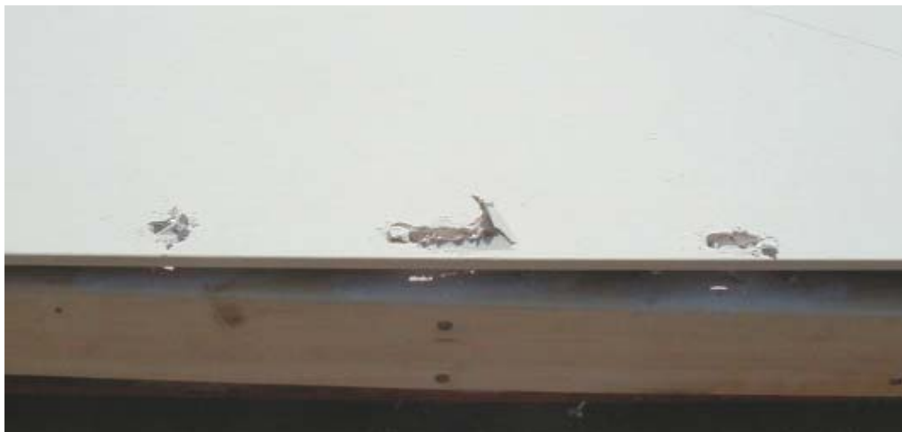
Figure 45: Gypsum nail rip-through along end stud
