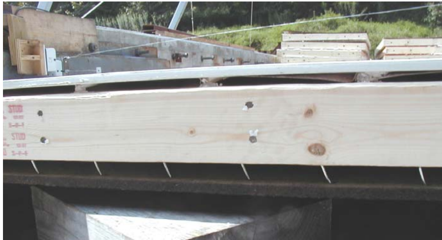
Figure 26: Nail pullout and tear-through of fiberboard and gypsum
