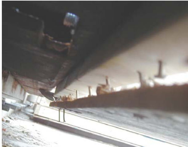
Figure 42: Sheathing nails unzipping along bottom plate of OSB
