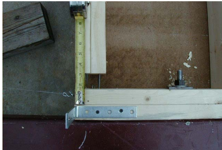
Figure 20: End stud separation at top of wall (hardboard)
