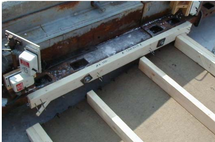
Figure 56: Wall separated from bottom plate after failure
