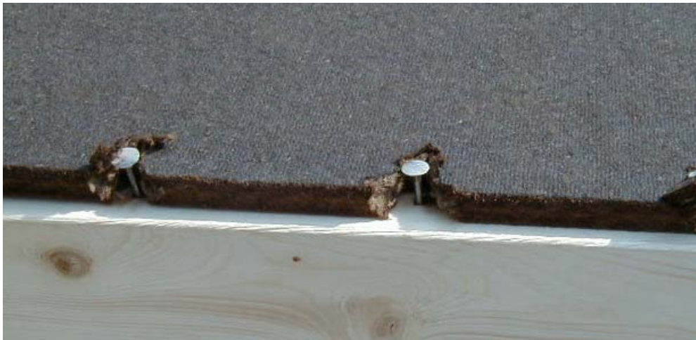
Figure 44: Nail tore-through in fiberboard panels
