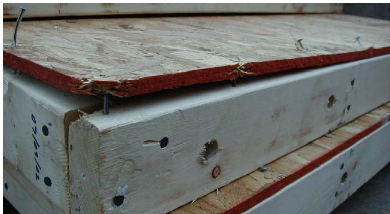
Figure 16: Nail pullout and tear-through on bottom plate (OSB)
